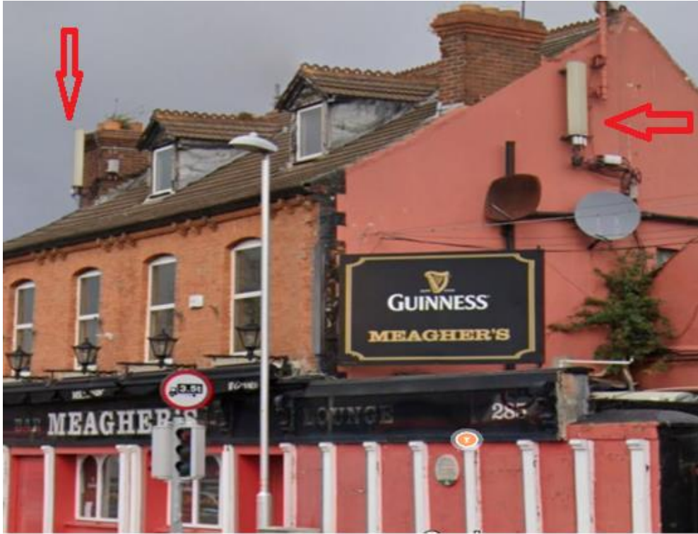
Meaghers Pub: Antenna attached to the front and side of building but not painted to match existing building walls.
