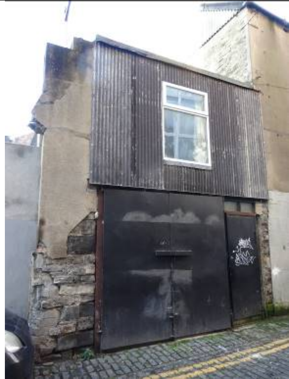
Fig.6: Two-storey mews building/warehouse fronting onto Jervis Lane Upper (known as both 56A Capel Street and 56 Jervis Lane Upper). Note the exposed sections of coursed calp limestone and brick masonry to lower level.
