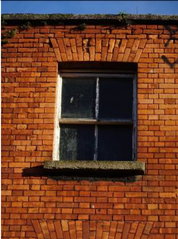
Fig.5: Detail of third floor window opening with granite cill and two-over-two timber sash window. Note the machine made brick to elevations laid in Flemish bond.
