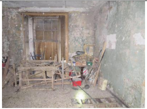
Figure 4 - Upper level rooms in poor condition and spoiled with pigeon droppings.
