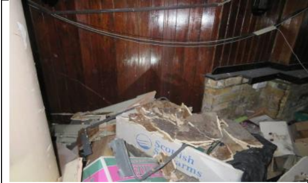
Figure 1 - Ceiling debris and previous tenant waste within public house.
