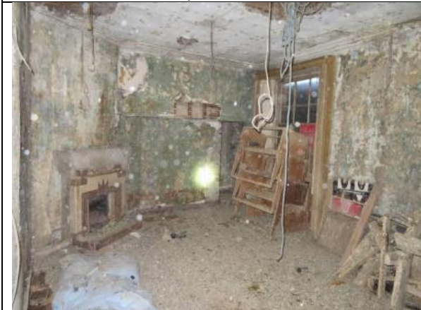
Figure 3 - Upper level rooms in poor condition and spoiled with pigeon droppings.
