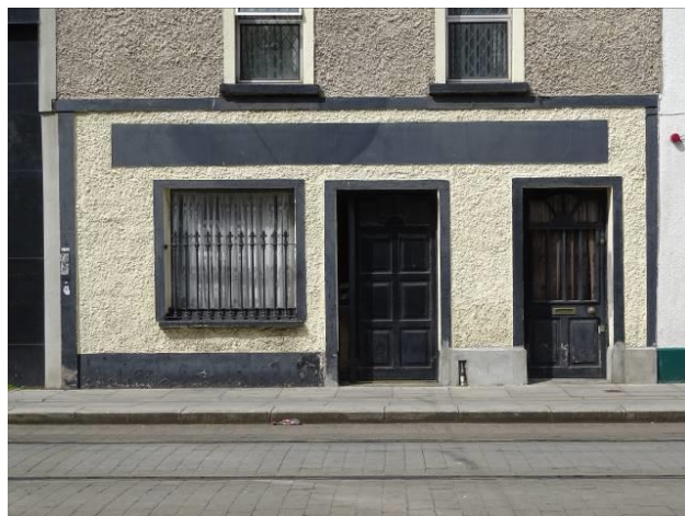
Fig.7: Detail of former shopfront to ground floor. Note the separate access to residential accommodation and rendered fascia board.
