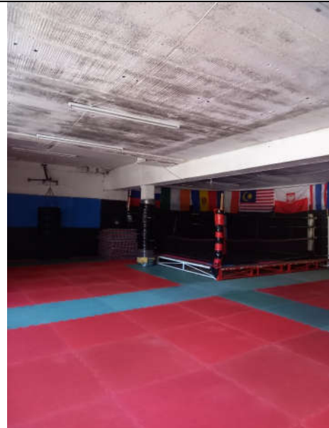
Fig. 5: Second floor interior showing concrete downstand beams to ceiling and modern finishes.
