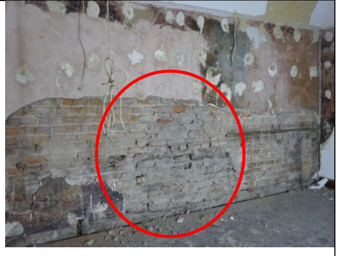
Fig. 8: Second Floor rear room of No. 10 with repaired brick work in the party wall to No. 11 as evidence of a 'creep hole' made during 1916
