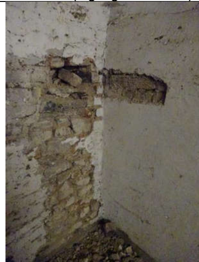
Fig. 10: Stripped plaster at 1 st floor SE corner with 19 th century brickwork and Calp stone, understood to relate to the former tenement at 4 Moore Place.
