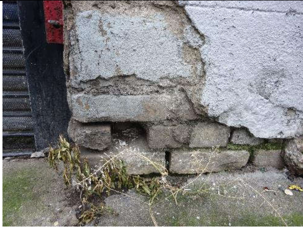
Fig. 5: Exposed section of stock brick dating from c.1920 at low level to the northeast corner of main Henry Place elevation.
