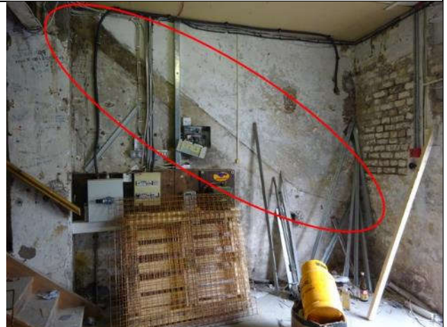
Fig.8: Scaring of former staircase to interior of the west elevation (highlighted in red).
