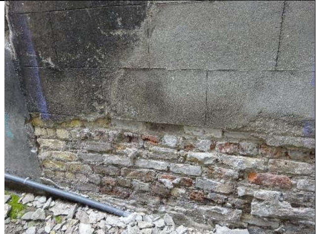
Fig. 6: Exposed section of early 19 th century red brick to the southern part of the east elevation, understood to relate to the tenement building at No. 4 Moore Place.
