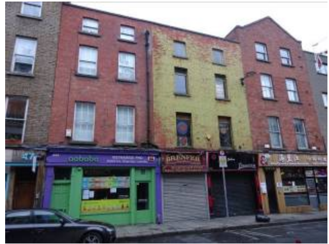
Fig. 4 Nos. 46a and 46/45a from east; note shared downpipe between the two properties
