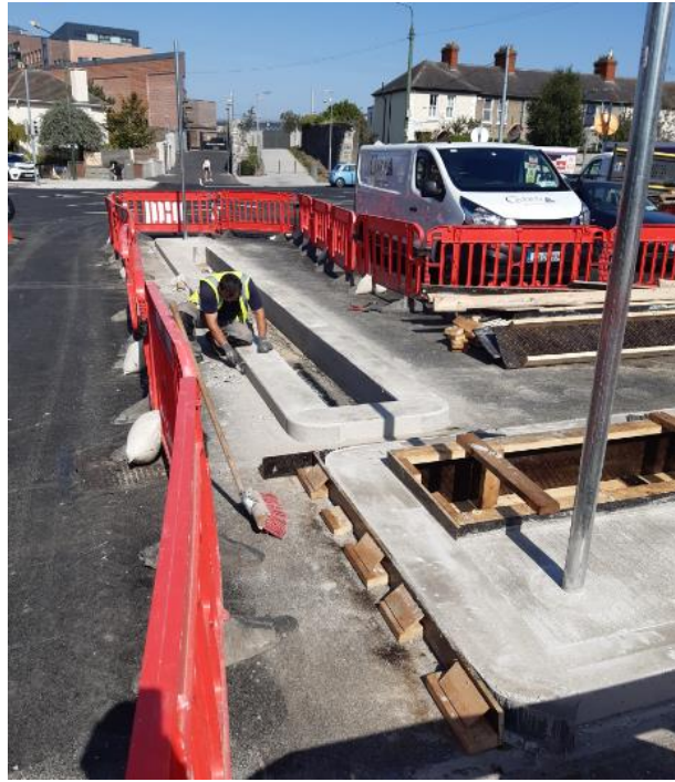
Construction underway on concrete buildouts with planting / landscaping at the filtered permeability location.
