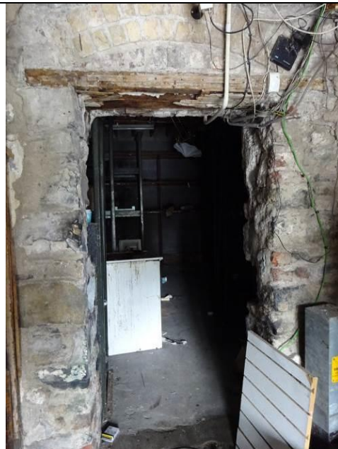
Fig.12: Rear door opening directly opposite main entrance lime washed with brick arch and remains of lath and plaster to timber lintel
