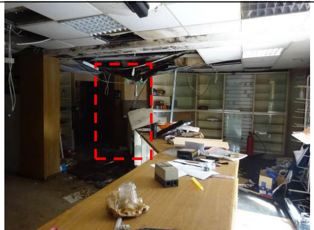
Fig.19: Ground floor shop looking north note angles of corner fireplace dashed in red
