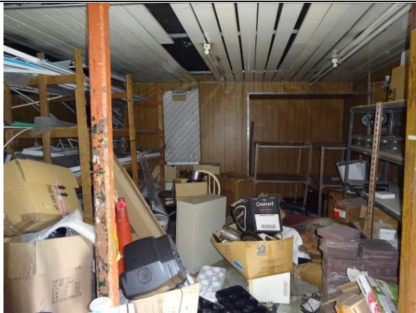
Fig.9: Open plan shop looking north with chamfered post supporting first floor internal walls and chimney stack in north wall
