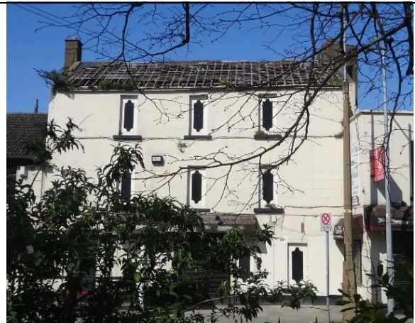
Fig.5: 152 Harold's Cross Road, natural slate stripped from front pitch
