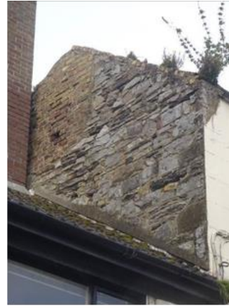
Fig.8: Rubble stone gable end to south with brick coursing to eaves and traces of an original brick chimneystack
