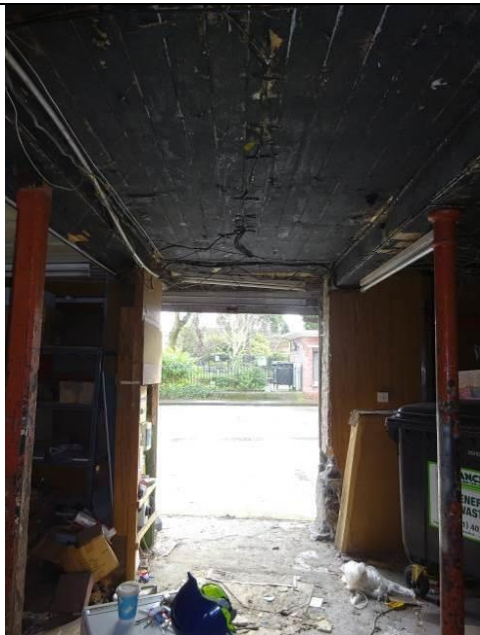
Fig.11: Main shop entrance flanked by cast and timber support pillars and timber beams above
