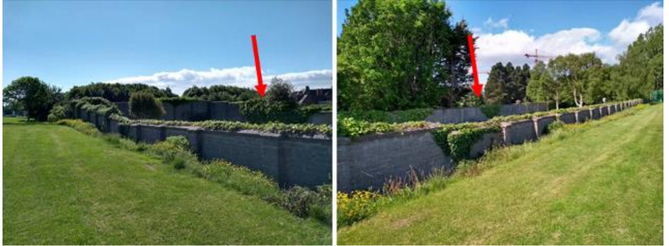
Wall has a modern render of pebble dash. No historic fabric was visible.
