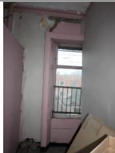
Fig 14: Surviving window joinery and cornice to rear wall at first floor; note partition cutting open
