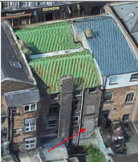
Fig 7: Rear elevation with blocked round-headed opening arrowed red to No. 46
