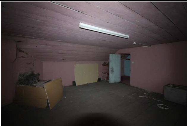
Fig 17: Third floor room to southeast corner looking west; note corner fireplace, timber to ceiling and early timber door
