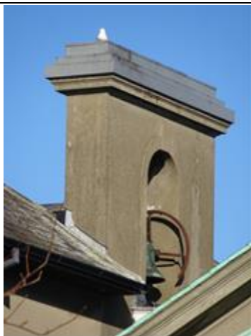
Fig.7: East chimney stack incorporating bellcote, housing a bronze bell with bell wheel.
