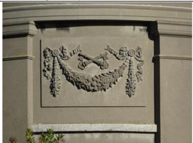
Fig.8: Decorative render panels incorporating swaged embellishments and the keys of Saint Peter.
