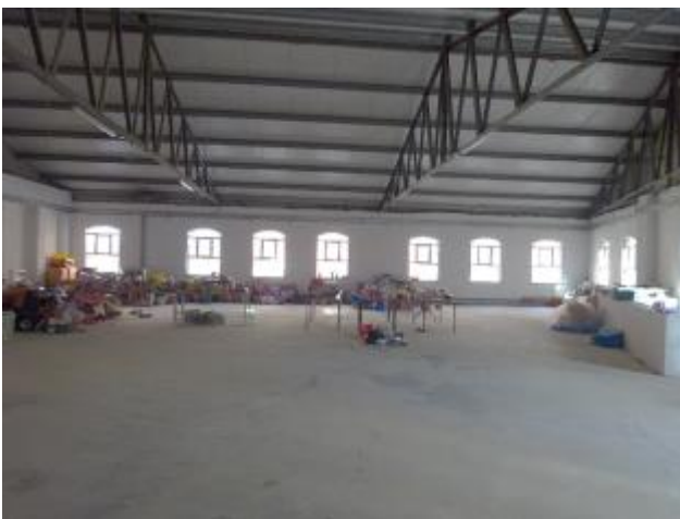
Fig 12: View of first floor, east end of building looking north; note recent roof structure and concrete floor
