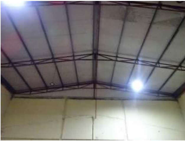
Fig 16: Roof and west wall of space to rear of east end of building
