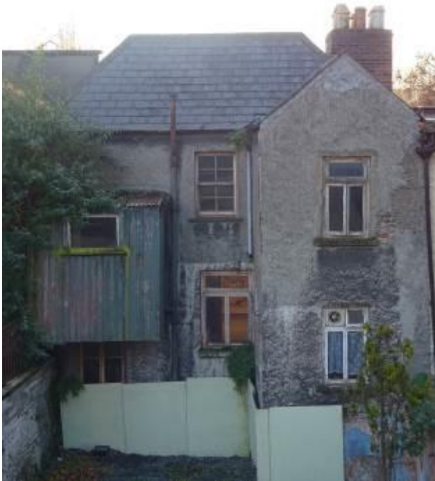
Fig.6: Rear/north elevation with steeply pitched roof and gabled closet return (indicative of an early date).
