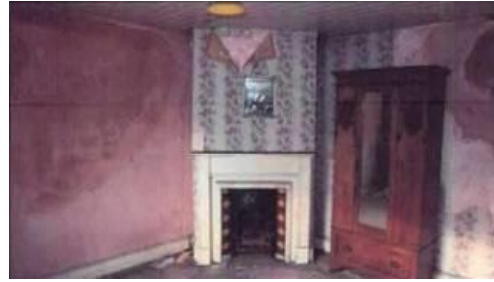
Fig.20: Aspect of second floor front room. Note the corner chimney breast with cast-iron fireplace.
