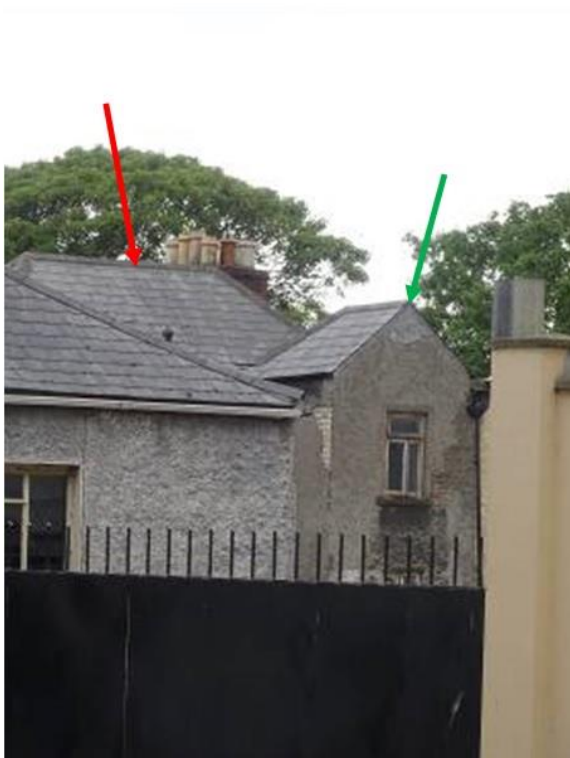
Fig.6: Rear aspect of steeply pitched double-hipped roof (arrowed red) and gabled closet return (arrowed green) indicative of an early date.
