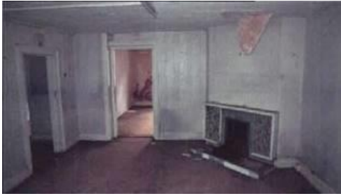
Fig.19: Aspect of first floor rear room. Note the low floor to ceiling heights, substantial corner chimney breast with late 20th century tiled fireplace and moulded architrave to doors.
