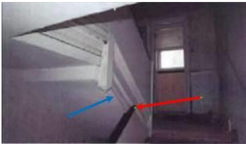
Fig.15: Detail of staircase between first and second floors. Note the intersecting handrail (arrowed red) and moulded closed string typical of the early-to-mid 18th century (arrowed blue).
