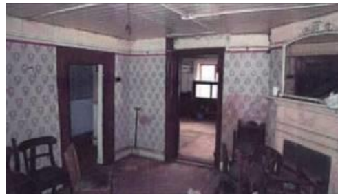
Fig.16: Aspect of ground floor rear room. Note the low floor to ceiling heights, substantial corner chimney breast with cast-iron fireplace and moulded architrave to doors.
