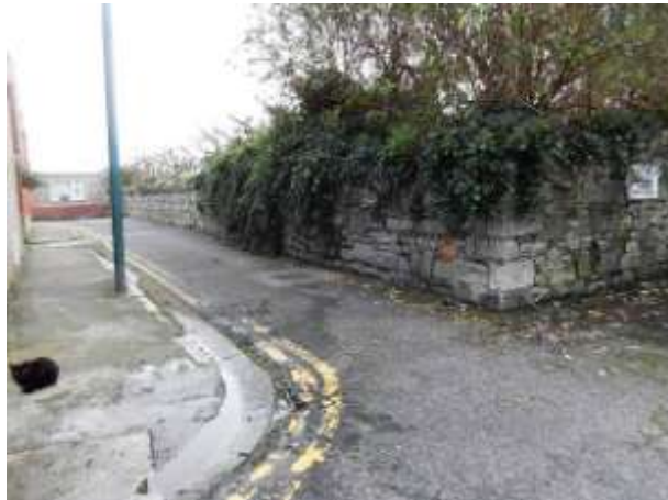
View of limestone calp wall at west end (boundary with rail line)
